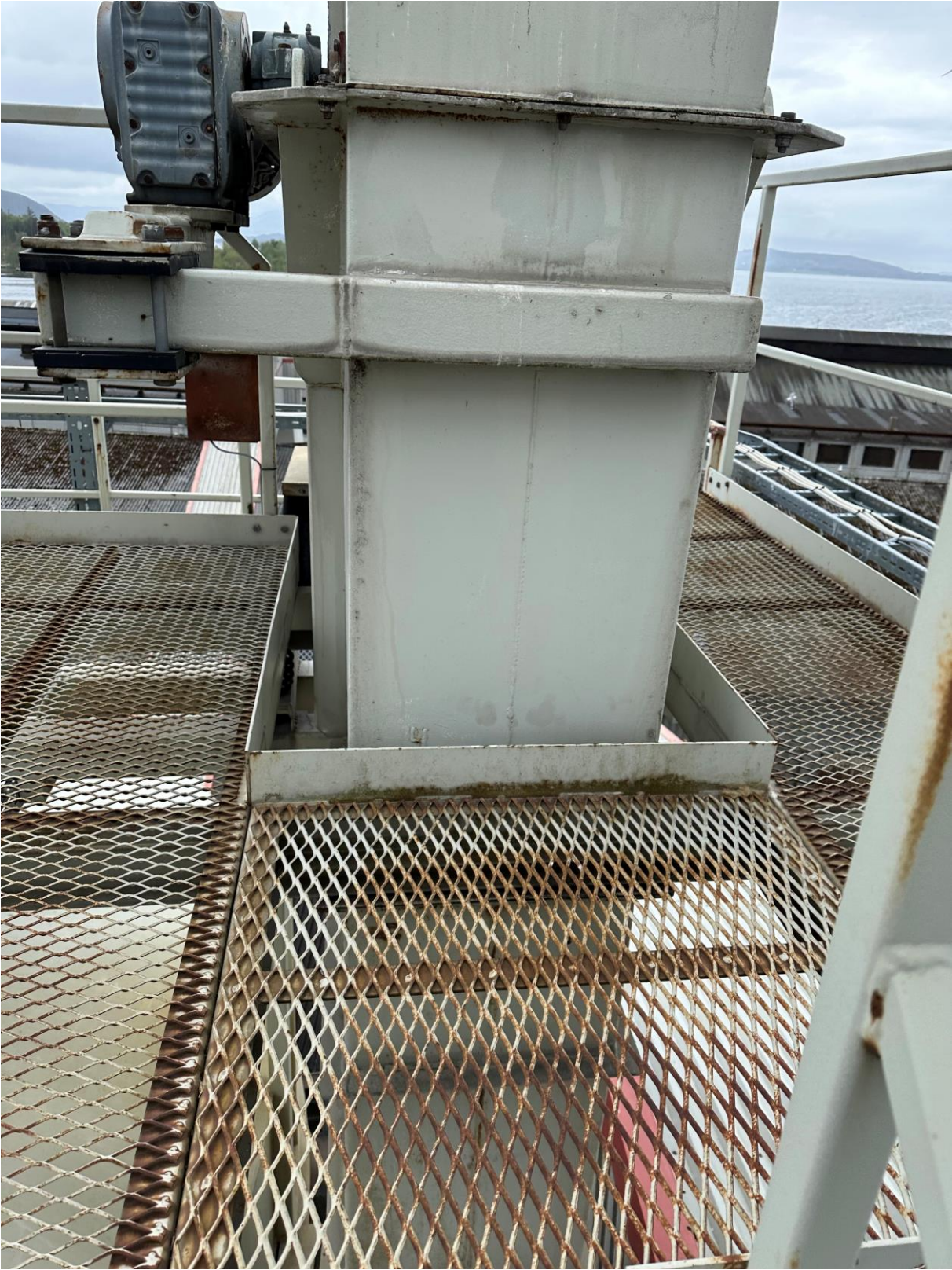
Elevator top over silo
